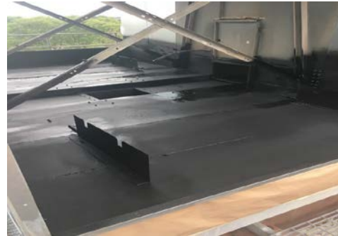
Freshly lined basin is now leak free and will provide years of extended life.
