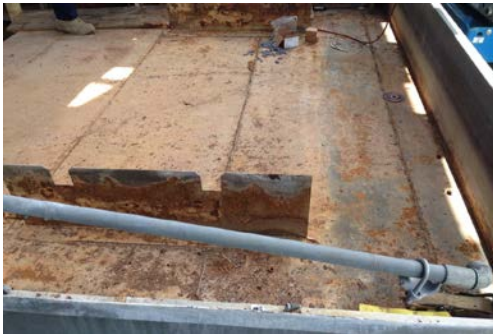
Rusted and leaking basin was at the end of its useful life and needed replacement.
